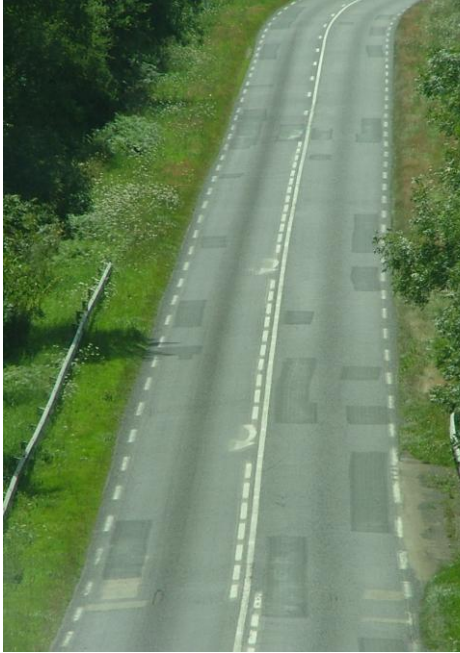
AC pavement exhibiting Chip Seal surface dressing maintenance throughout life up until total resurface dressing takes place.
